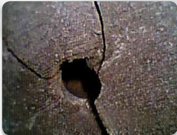
Using the optional Close-Focus Tip, fine cracks are detected inside a combustion chamber.
